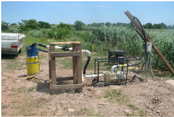
Above, a photo of SAI's variable speed high capacity pump.
