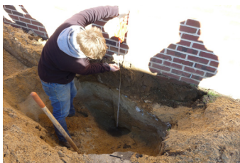
SAI Field Scientist Jack Taylor performs geotechnical sampling for the NJSDA project.
