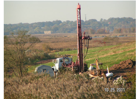
A view of an extraction well at ILR Landfill, with wetlands in the background. This area will be used to site some of the solar panels when the project is completed.
