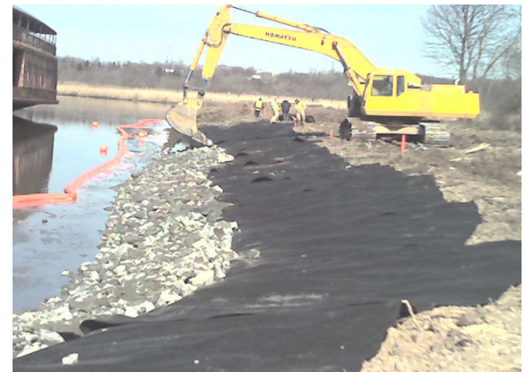
...and as it can be seen today, under construction to restore the riverbank. Photographs copyright Sadat Associates, Inc.
